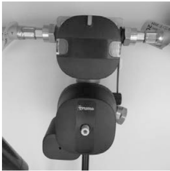
Fig. 71: Gas supply (with Eis-Ex and remote control)
