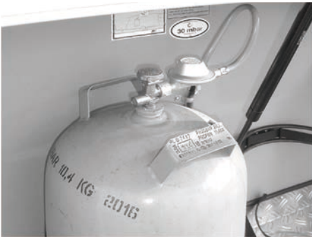
Fig. 70: Gas bottle with low pressure regulator and low pressure hose
