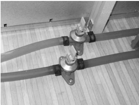
Fig. 97: Drain valves opened
