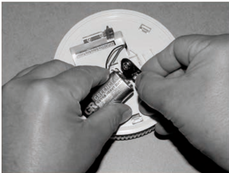
Fig. 228: Replacing the block battery
