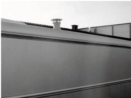
Fig. 77: Exhaust gas stack of the gas heater
