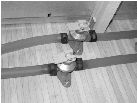
Fig. 171: Closed drain valves
