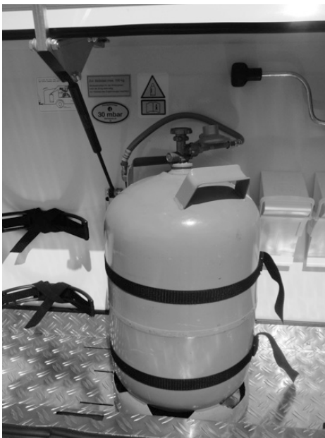
Fig. 80: Open gas locker
