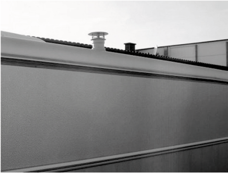
Fig. 89: Exhaust gas stack of the gas heater
